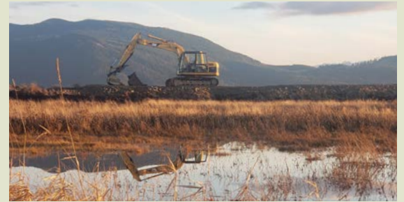
King tides showed the age of the private dike. Trust staff met with community partners to begin talks on solutions to the aged dike.
